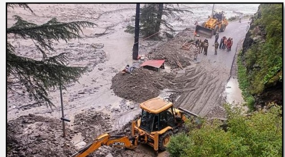
Retiro de escombros en caminos cerca de Harsil, Uttarkashi /Debris removal on roads near Harsil, Uttarkashi Foto/Source: PTI
