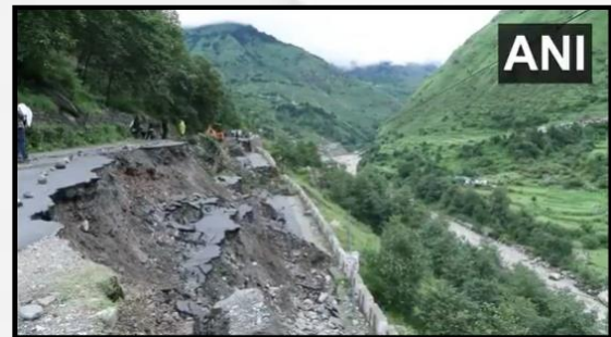
Carretera dañada en Bhatwari Uttarkashi / Road damaged in Bhatwari, Uttarkashi Foto/Source: @ANI
