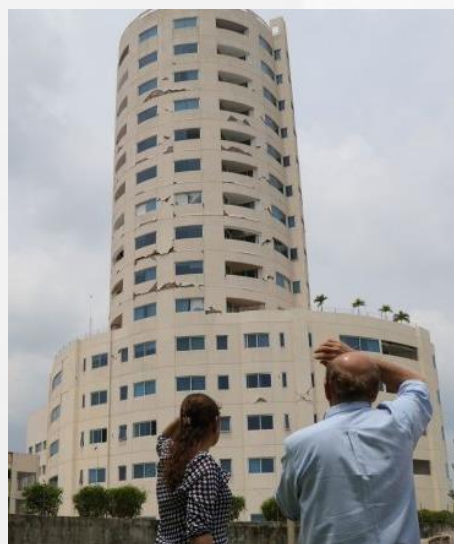
Daños en Torre Zafiro, Tabasco Damage in Zafiro Tower, Tabasco
